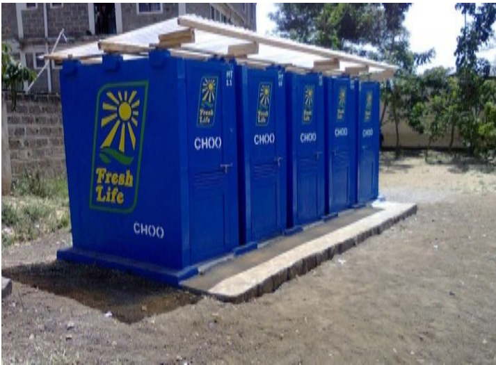
Privately delivered Sanergy Fresh Life toilets
