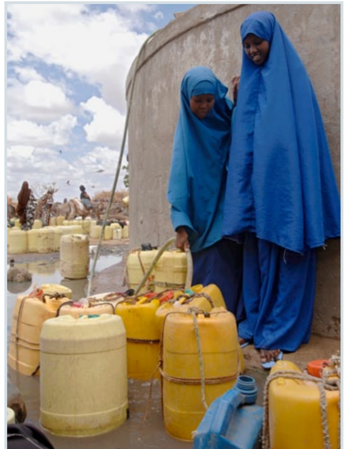
This borehole in Goriale Location was built by the Government but fell into disuse in the early 2000s. CARE approved the repair of the borehole and it now supplies 1,440 households with clean water for their family and animals. Due to the severity of the drought, however, the surrounding desert area is littered with the carcasses of many animals.
